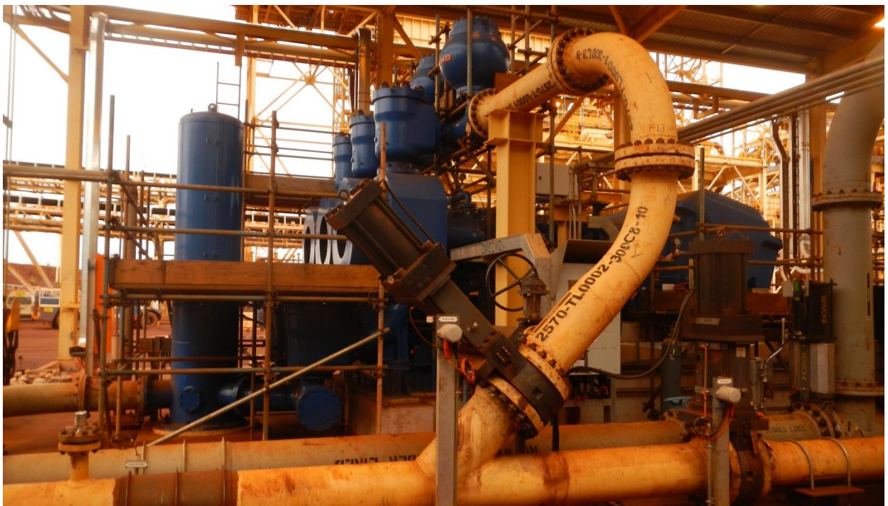
Delta ASME Class 600 slurry knife gate on PD Pump circuit
