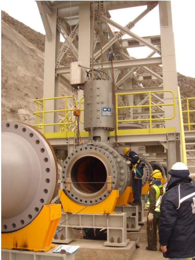
High solids slurry isolation ball valve in a copper concentrate pipeline
